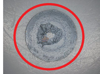
The contact part is discolored to black due to sulfurization
